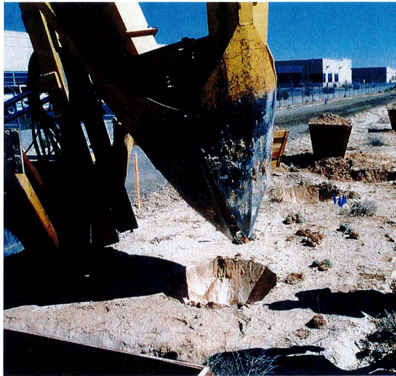
Figure 3.2-1. Salvaging a Las Vegas bearpoppy plant at the North Las Vegas Airport with a tree spade.
