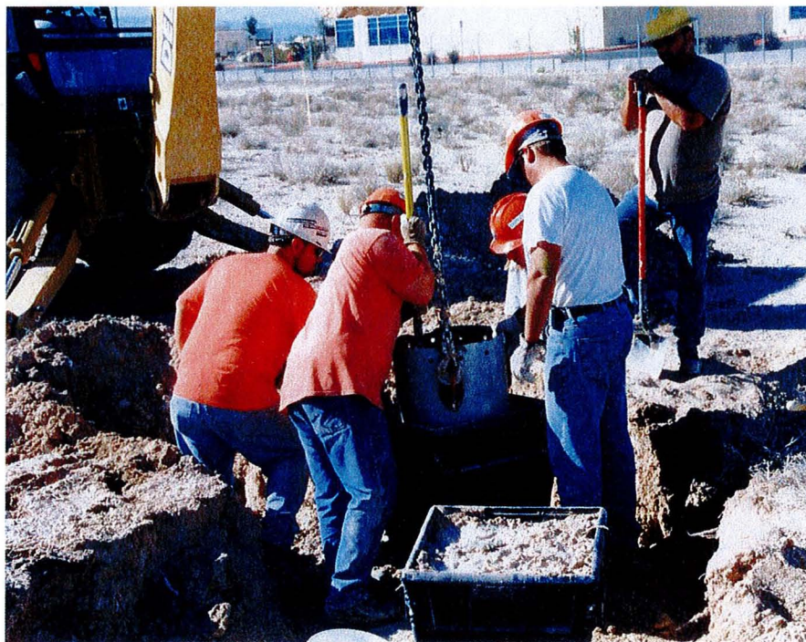
Figure 3.2-3. Salvaging a Las Vegas bearpoppy plant at the North Las Vegas Airport with the pipe method.
